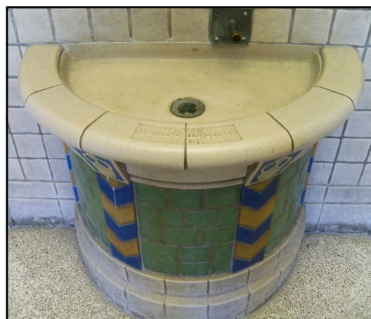
Figure 17. The present condition of the fountain's basin showing the dedication tiles and the capped plumbing.
